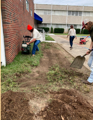
Figure 2: Students removed the existing sod from the landscaping site and placed it on the west side of the building in the hopes it would grow there come springtime. (Photo by Paul Jackson. October 26, 2020.)
